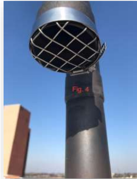
Figure 4. Example of the proper size of the wire mesh cover installed on the chamber exhaust pipe; free of potential occlusions.
