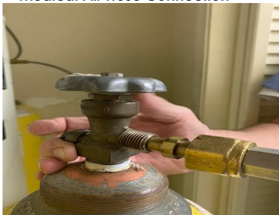
Outlet Valve too Small for Medical Air Hose Connection
